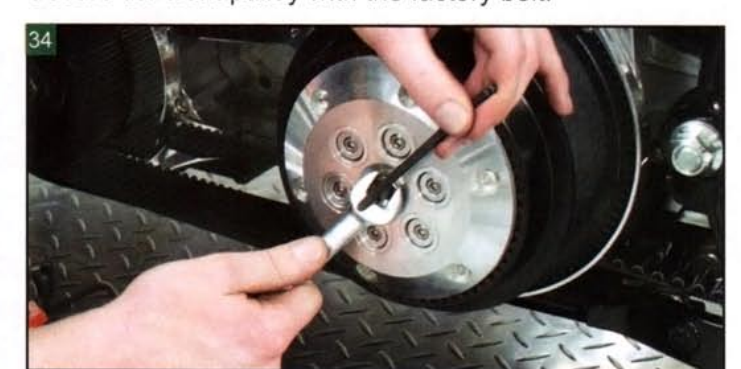
Collapse the clutch cable adjuster and adjust the clutch by turning the set screw until it touches the transmission push rod, then back off 1/2 turn and set the locking nut.
